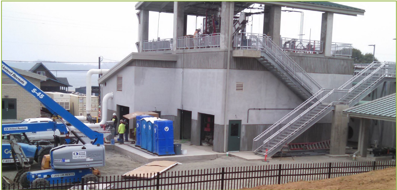
Coos Bay water treatment facility. Photo credit: Oregon DEQ
