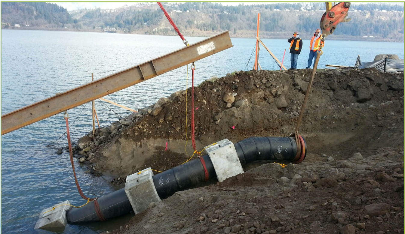
Installation of a sewer outfall pipe. Photo credit: City of Hood River
