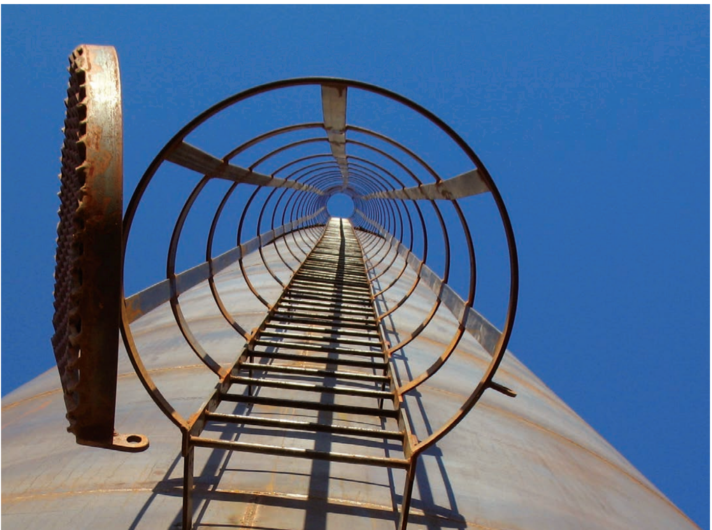
Logan County Rural Water District # 2- Stand pipe.
