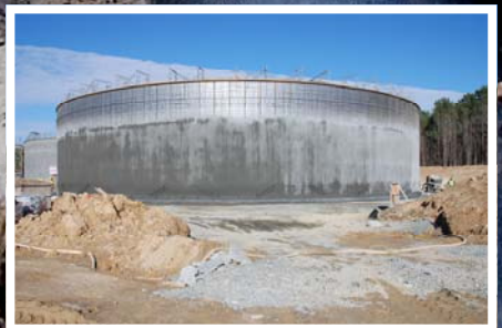
Construction that is part of the South Granville Water and Sewer Authority Wastewater Treatment Plant (CS370925-02)
