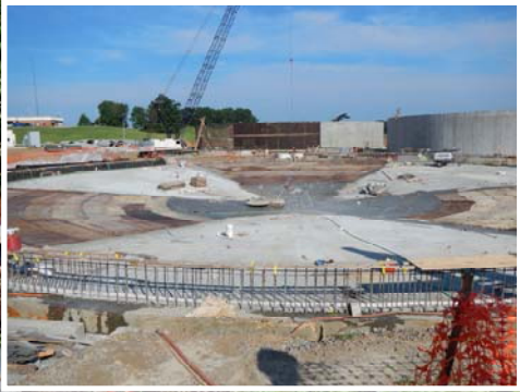
Construction at the Neuse River WWTTP for the City of Raleigh (CS370419-18)
