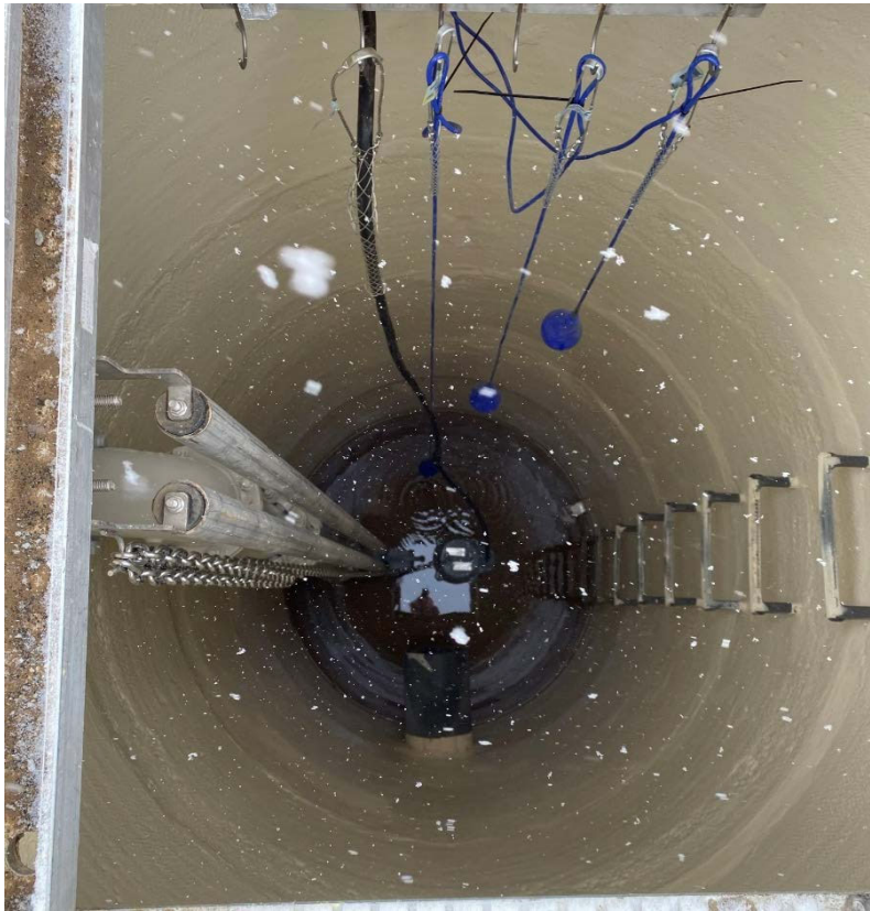
City of Grants CWSRF 077 Pump Station with Snow
