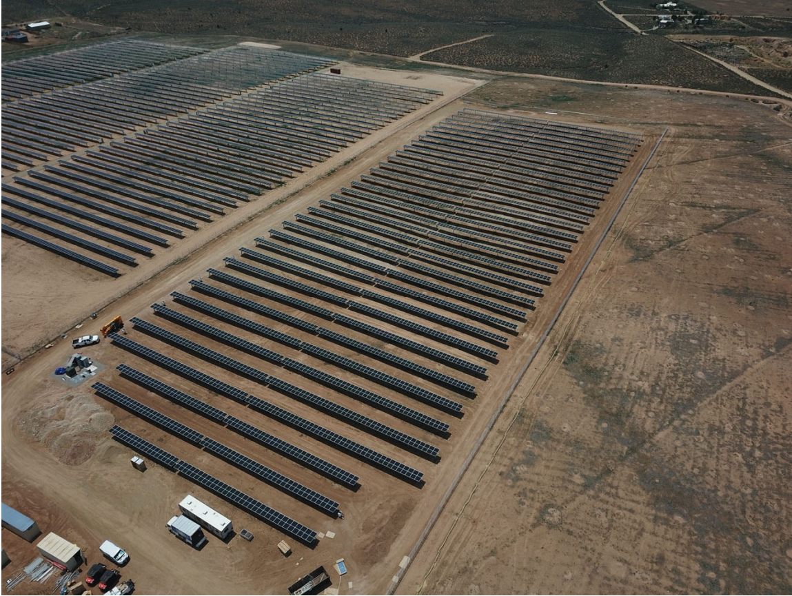
The Village of Taos WWTP Solar Array CWSRF 053
