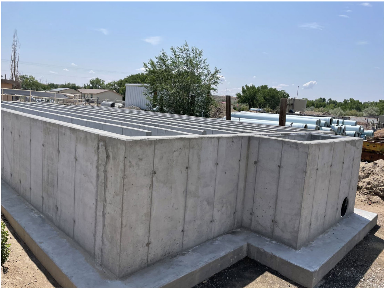
The City of Bloomfield CWSRF 103 Chlorine Contact Chamber
