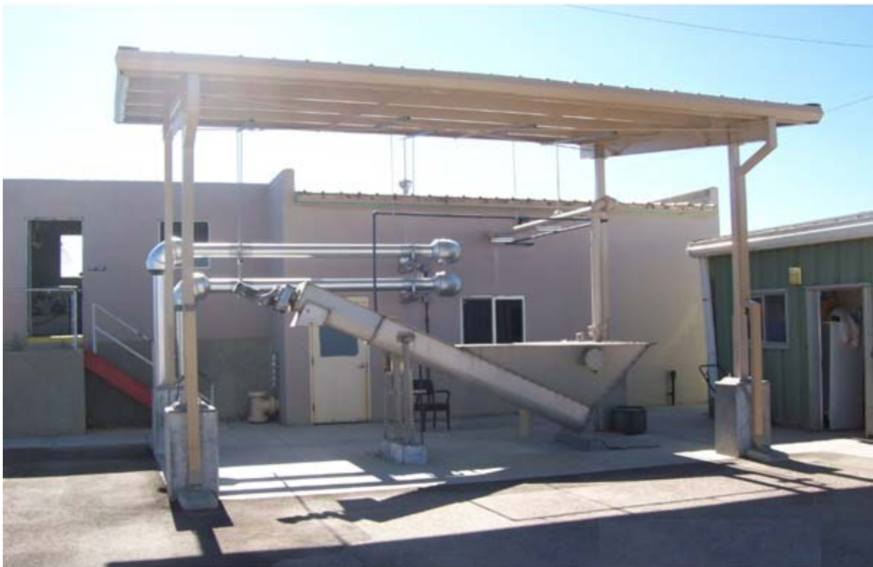
City of Gallup Grit Classifier at Headworks
