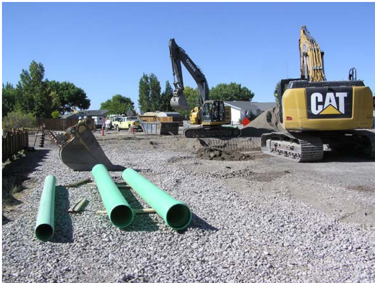
Churchill County System Improvements
