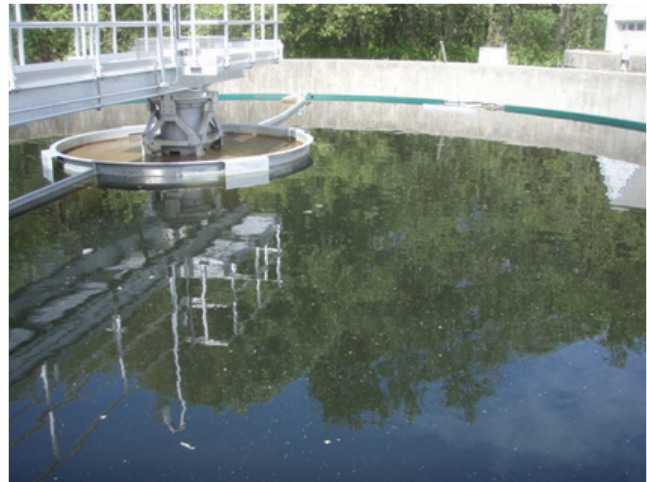
Letchworth Avenue Wastewater Treatment Facility Billerica, MA
