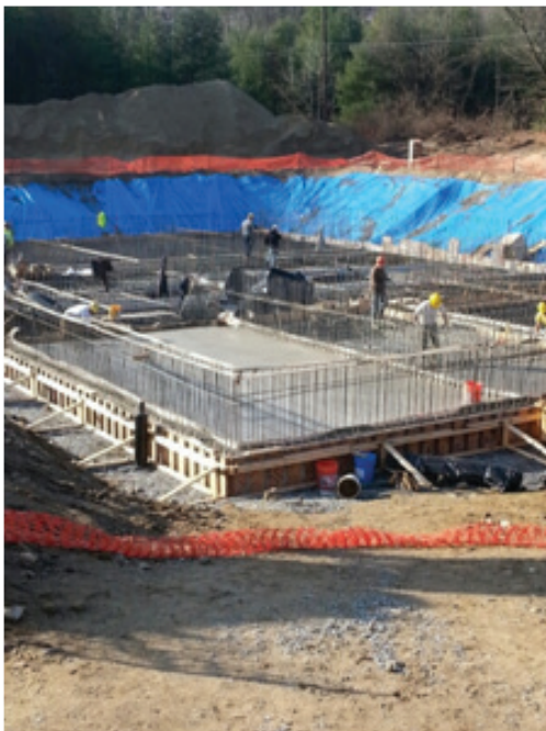
Acton Water Treatment Facility
