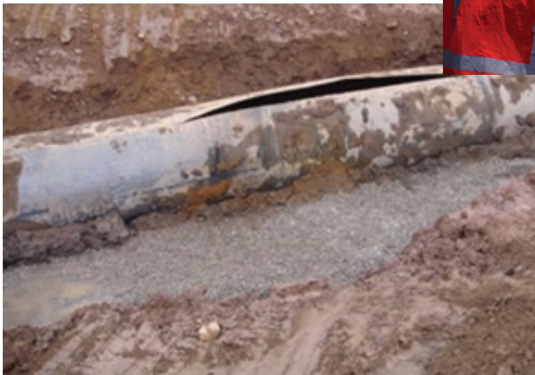
Ruptured Water Transmission Main
