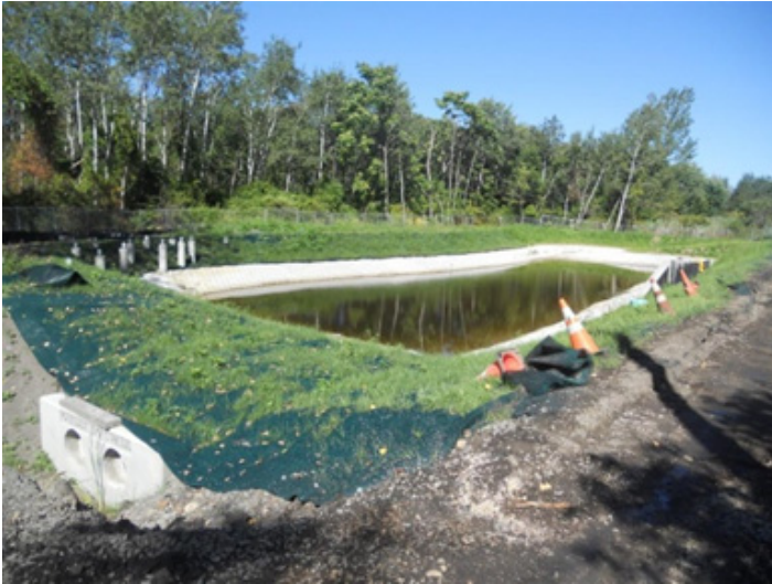
Stormwater Treatment System
