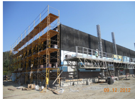
Tertiary Treatment Building N. Attleborough
