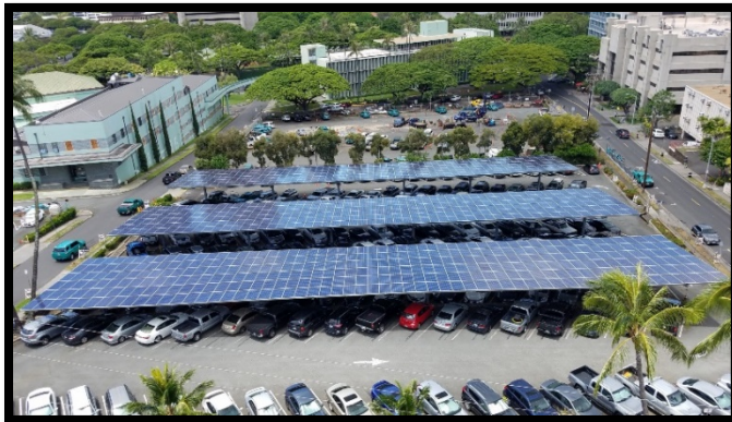
▲ PV panels installed in the parking lot of the Beretania station
