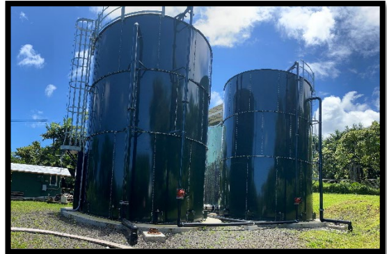
▲ New 50,000-gallon tanks
