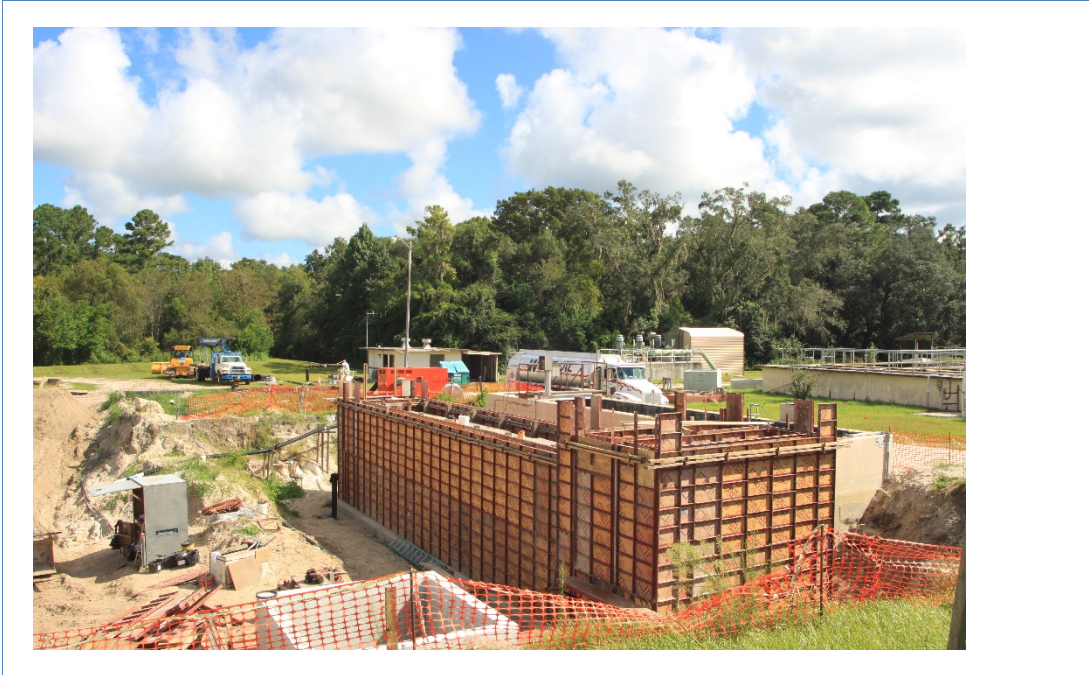
Perry Wastewater Treatment Plant
